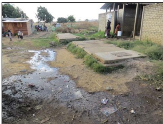
Burst sewer pipe close to the ablution block
