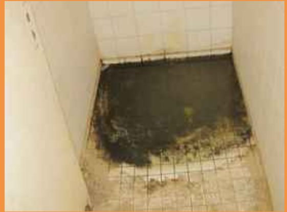
A broken and blocked shower
