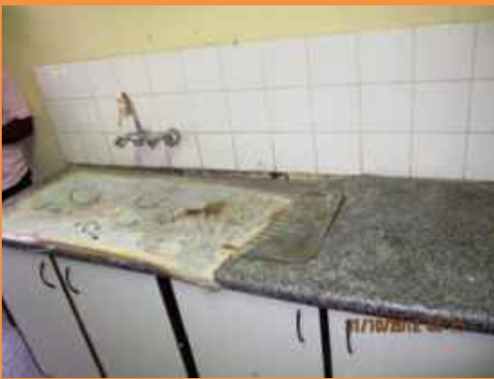
A broken sink
